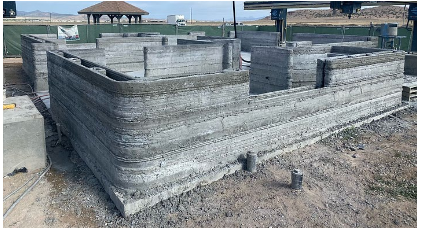
A 3D printed house at Yavapai College's Chino Valley Agribusiness Center. (Matt Mintzmyer/Courtesy)
