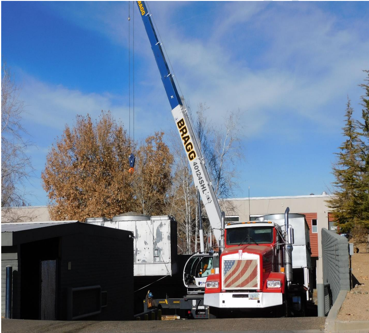
Removal of the heat exchanger as part of Building 1 boiler plant decommissioning
