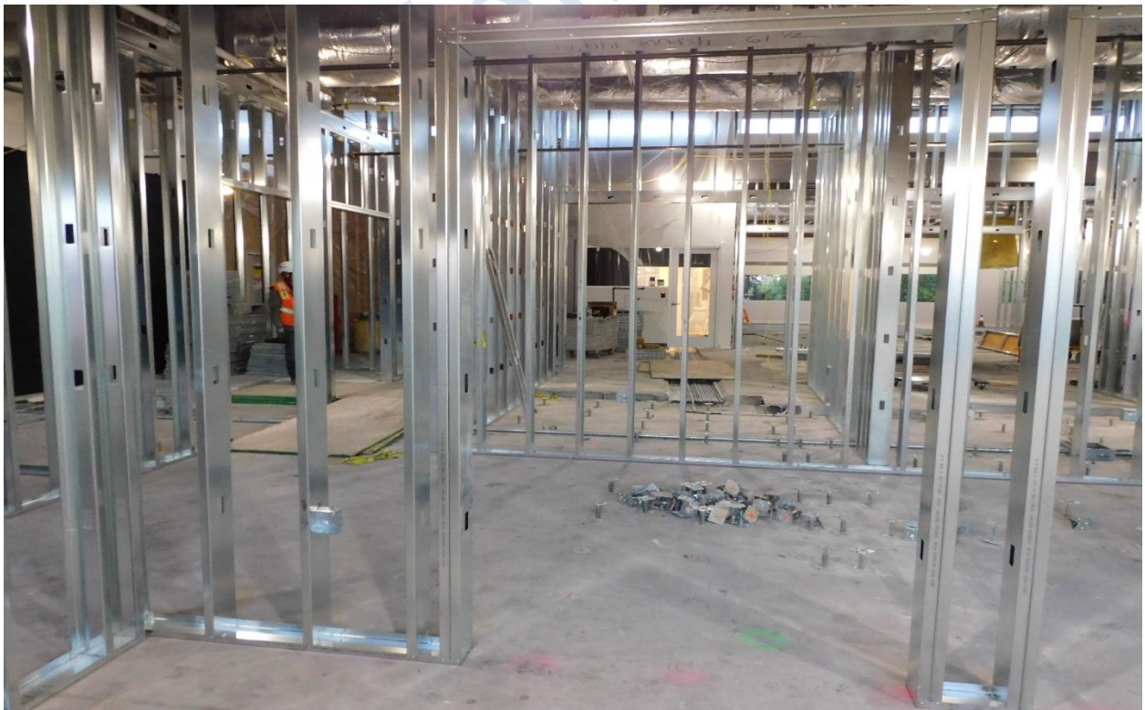
Framing and data cabling for One Button Studios and TeLS on the second floor
