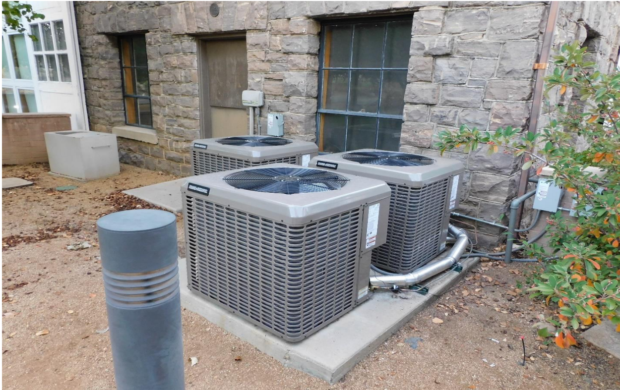
New Rock House A/C units
