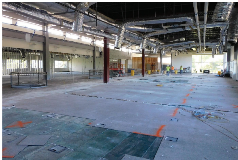
Construction for the Center for Learning & Innovation on the Prescott Campus, second floor.
