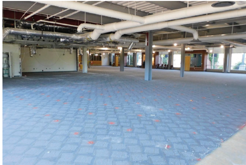
Construction underway for the Center for Learning & Innovation on the Prescott Campus, first floor.
