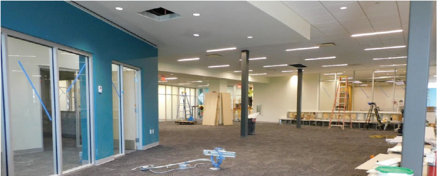
Construction in progress for the Center for Learning & Innovation on the Verde Valley Campus.
